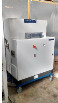
Electrical Power bay (for motors) and acquisition bay
